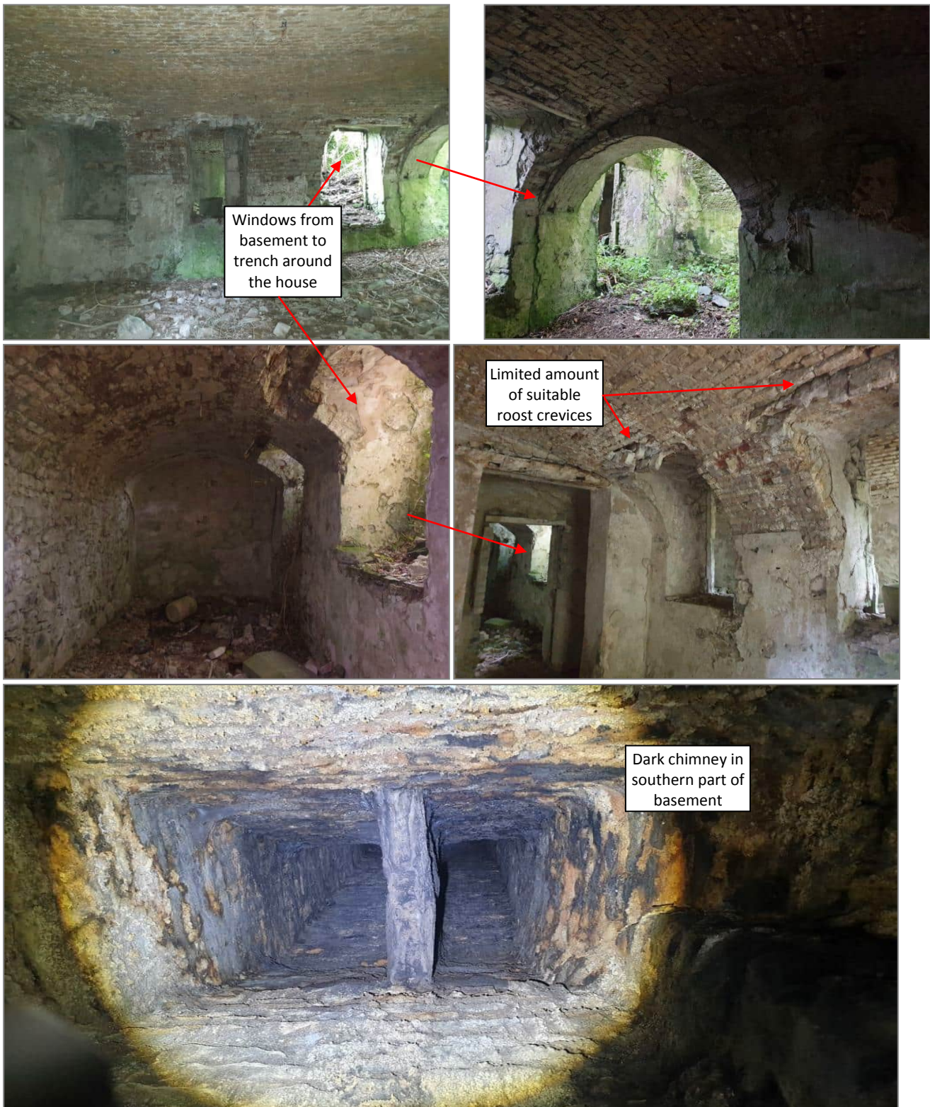
Plate 24. Basement area to the south of the ruins had daylight ingress through windows to a trench surrounding the house and through missing floors/ceilings over the basement. There were also limited suitable roost crevices in the brickwork ceiling of this part of the basement. There was a chimney in this part of the basement (bottom photo) where bats could potentially roost in darkness. There was only a very sparse scatter of old bat droppings in this area.
