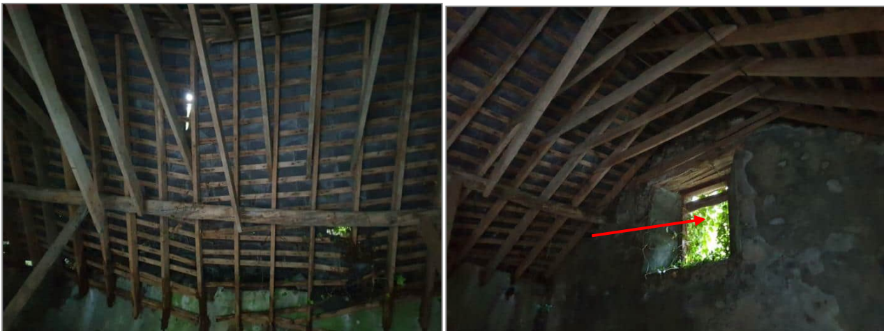
Plate 12. Collapsing slate roof, holes in roof and open window where one Soprano Pipistrelle emerged
