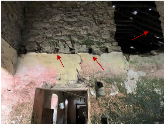
Plate 3-9: Potential roosting spaces in gaps created by missing roof beams and also on timber roof beams
