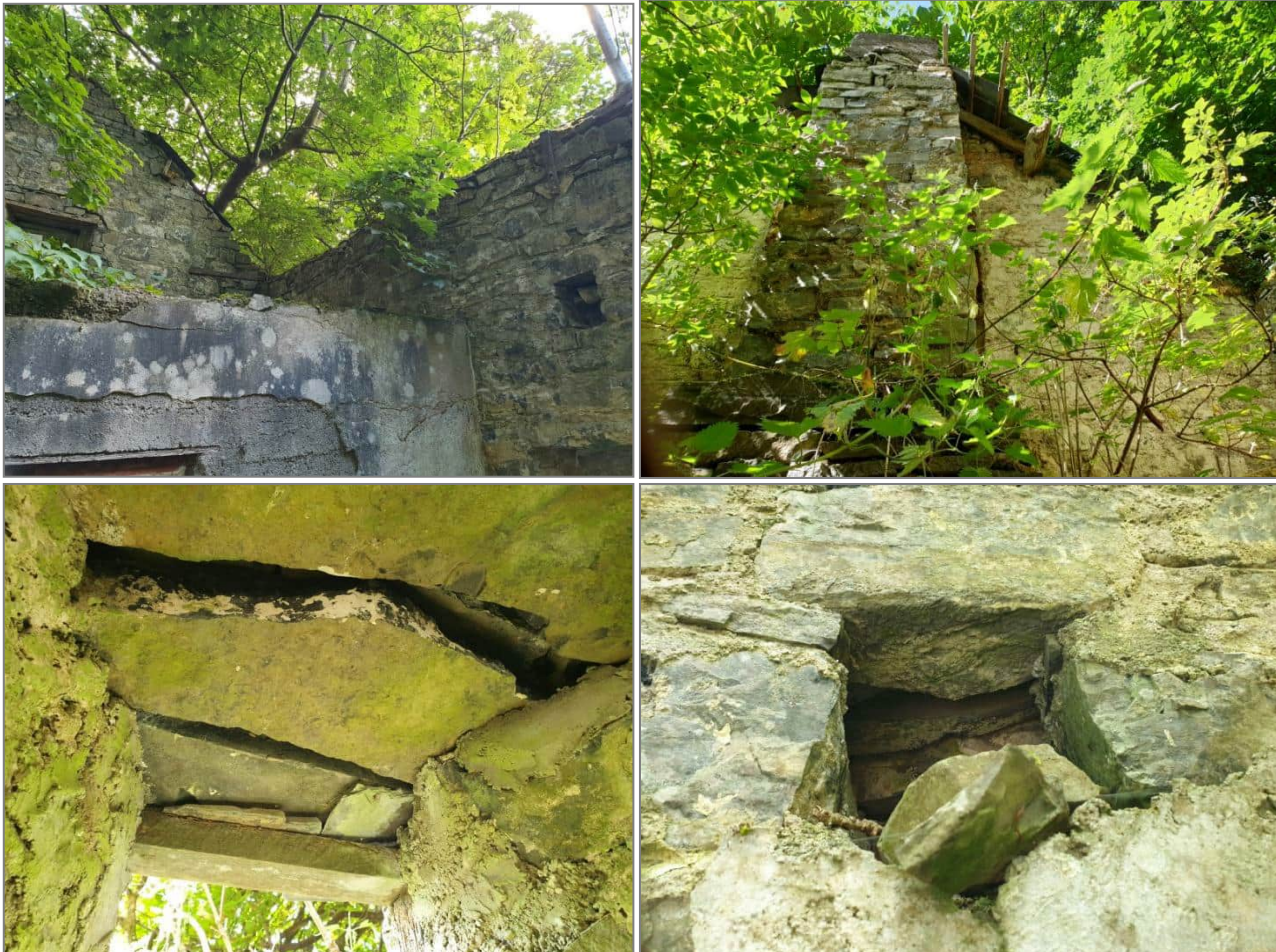
Plate 6. Some potential roost cracks and crevices in stonework at the old cottage ruin
