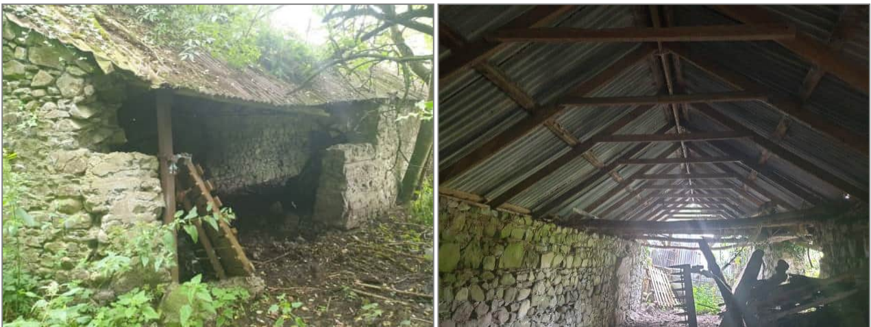
Plate 14. Stone shed with large openings in walls and corrugated iron roof had low bat roost potential
