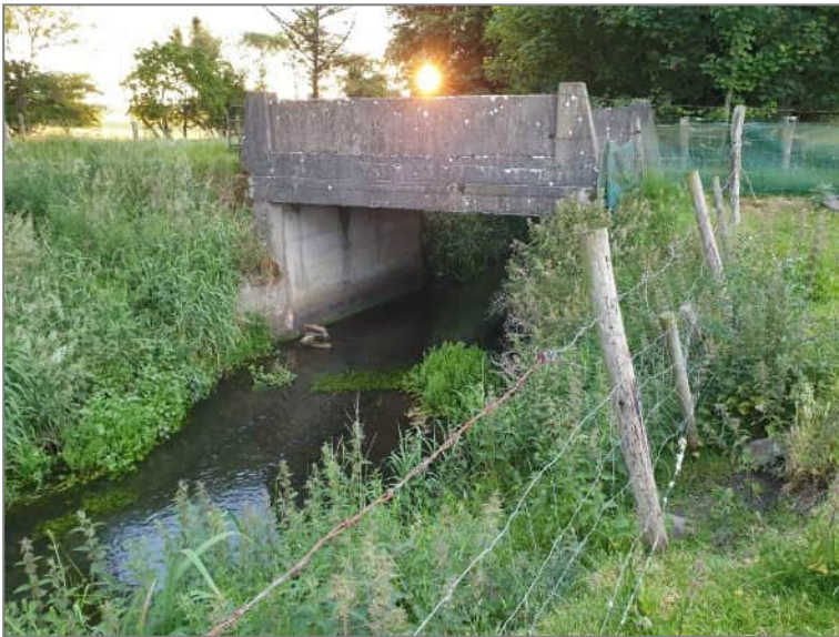
Plate 29. Negligible bat roost potential in this concrete bridge near Rosmead House ruins
