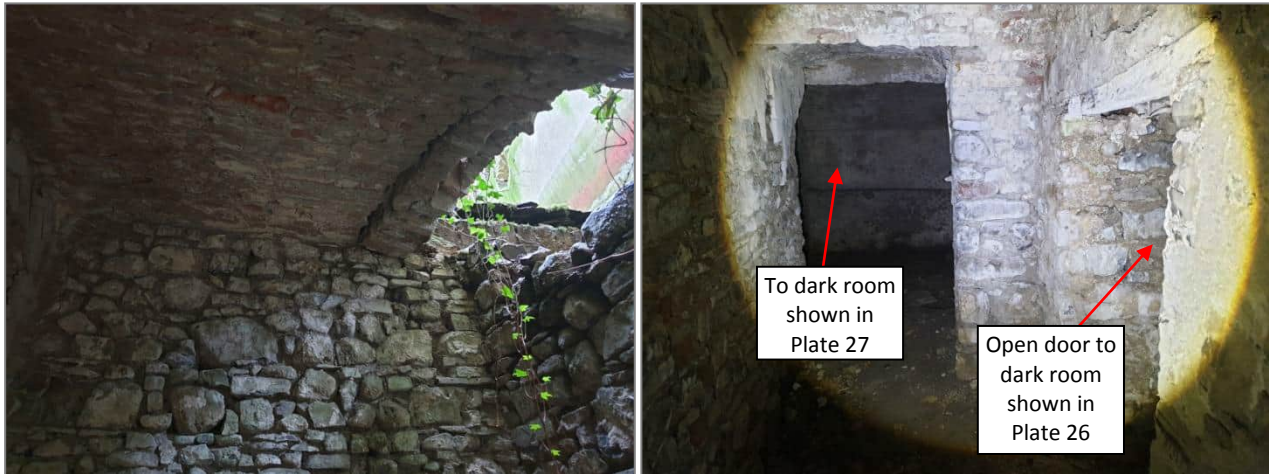
Plate 25. Open passageways and doors leading to dark rooms in the basement, as shown in Plate 26 and Plate 27
