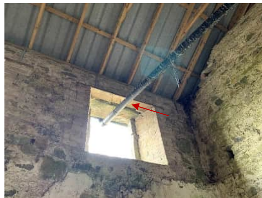
Plate 3-8: Potential roosting space between timber and stonework
