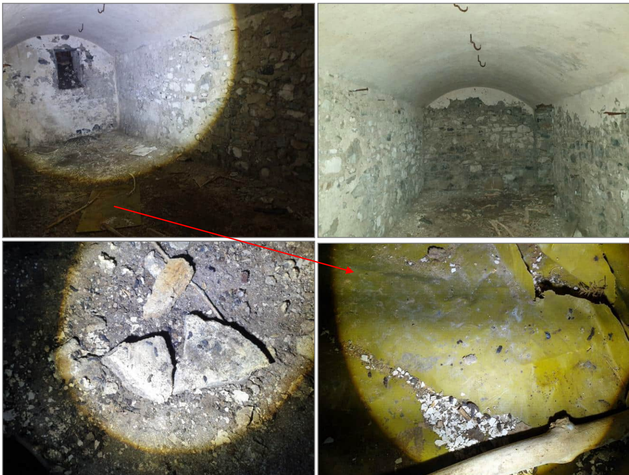
Plate 26. A dark basement room, which had sparse bat droppings and feeding remains of Brown Long-eared Bat and another unknown bat species on the floor. However, note the lack of suitable roosting crevices in the arched ceiling or in the stonework of the walls.
