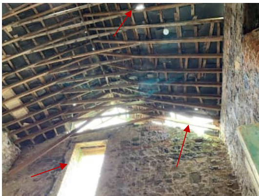
Plate 3-7: Potential access points in gaps between roof slates and missing windows
