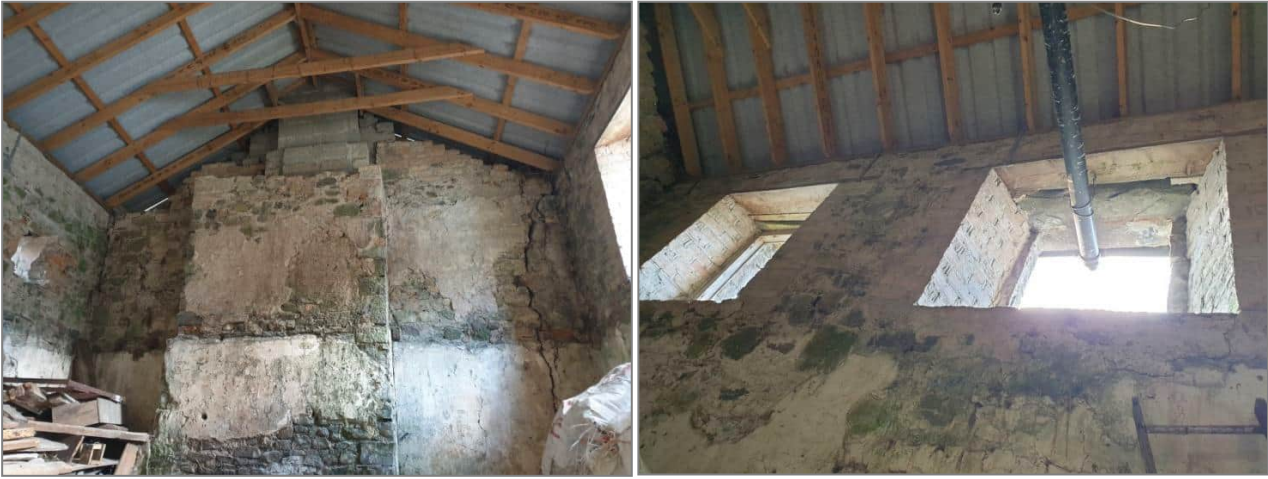
Plate 20. Cracks and crevices in stonework/bricks and gaps in window lintels offer bat roost potential
