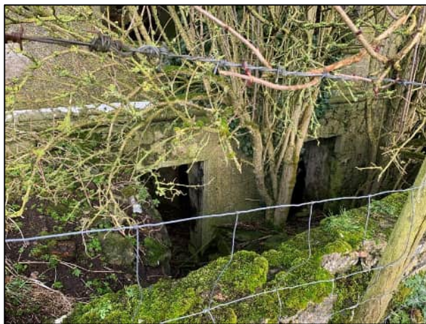
Plate 3-5: Lower level floor of derelict building
