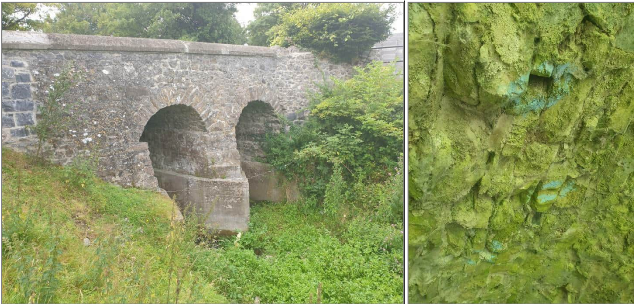
Plate 9. Double arch stone bridge over Stonyford River with potential bat roost crevices
